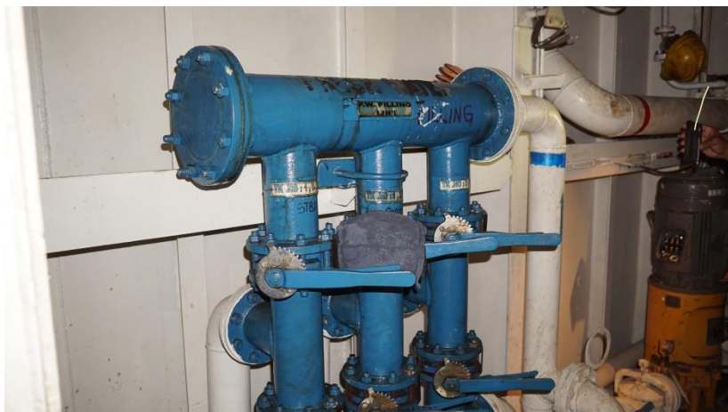
F.W Manifolds and Pumps
