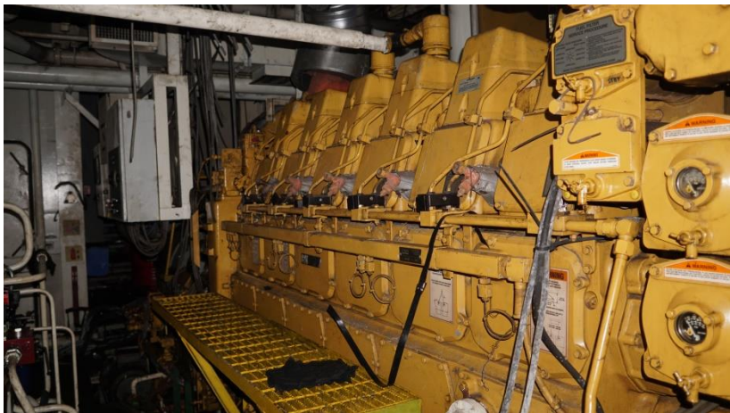
Portside Main Engine
