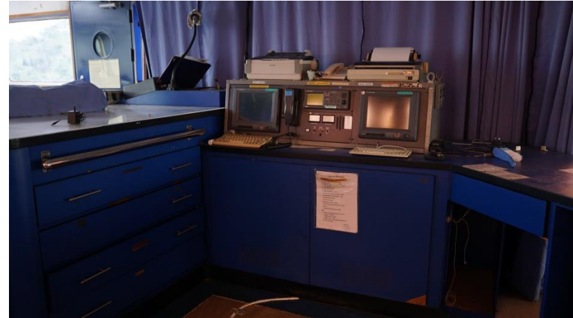
GMDSS Radio Terminal
